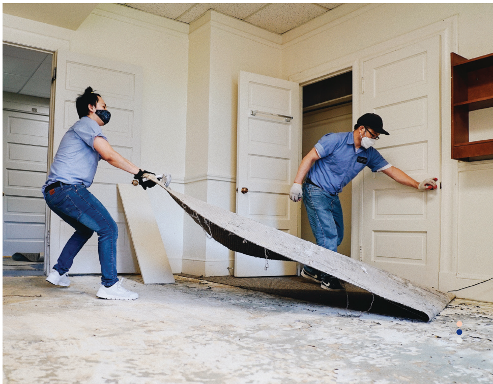
ABOVE: Renovation of Fort Worth Hall, the oldest building in Southern Baptist theological education still in use, will be completed in time for the fall semester.
